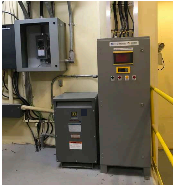
Illustration 3: HRG control panel powered with the RCMS490 & NGRM700 relays inside
