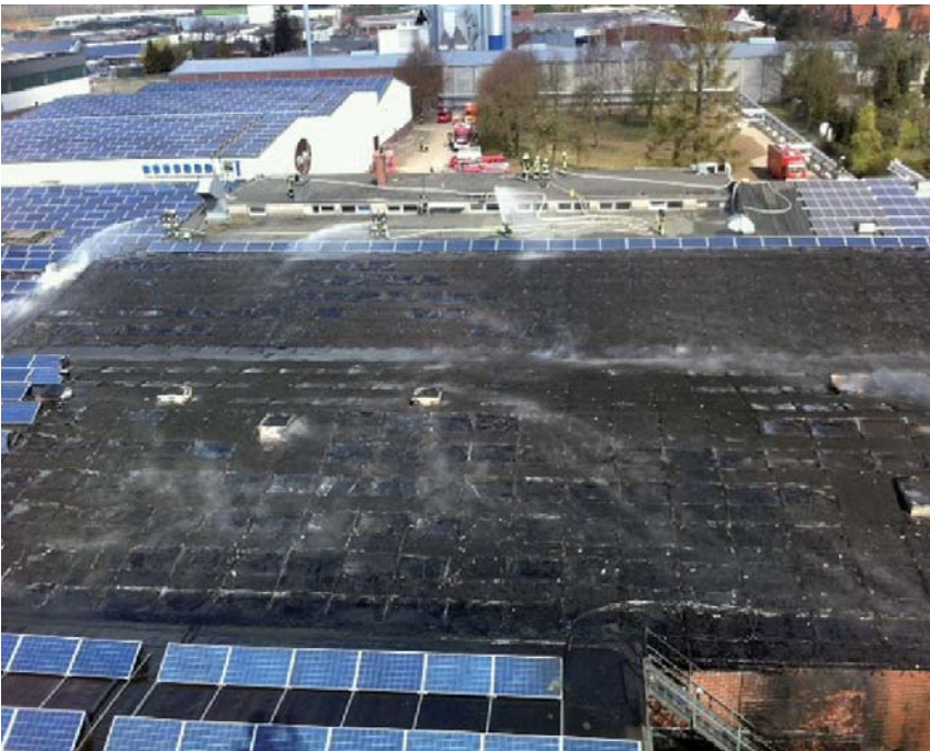
Fire safety: Rooftop PV system destroyed by a fire
