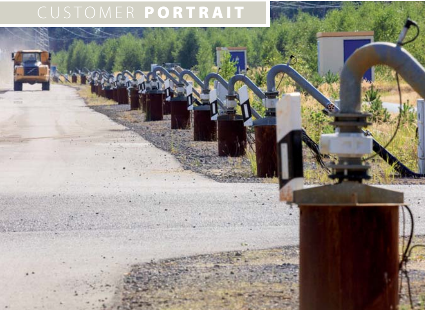
20 to 30 drainage wells – out of 2,000 in total – are supplied with energy by a transformer station (with blue door in background).
